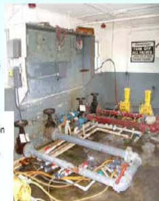
5S in Valve Room helps ensure correct application and delivery of feed
